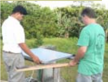
Ermain Requena and Mark Miller installing the Solar Panel at Pueblo Viejo Primary School
