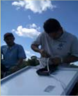
Plenty Field Officer Abib Palma work to install the Solar Panel in Corazon Creek Village
