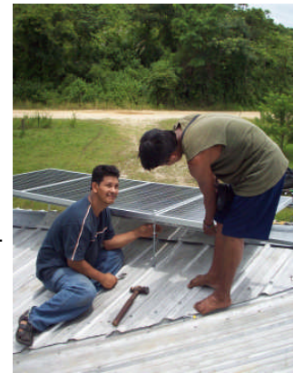
Abib Palma and RBNP Ranger installing solar panels on the visitor center roof
